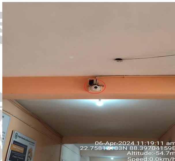
CCTV In Corridors
